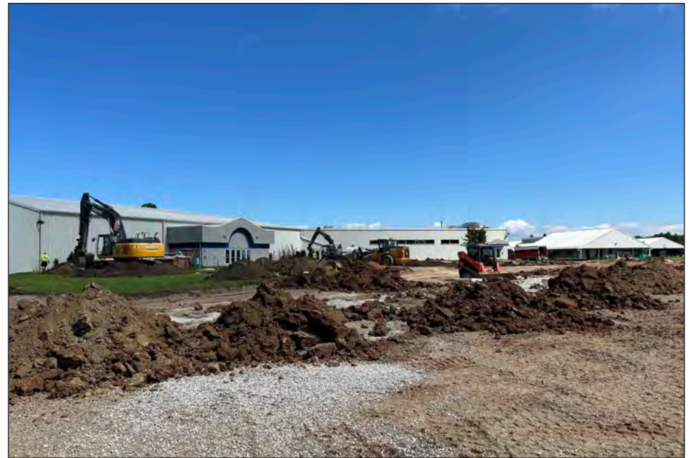
Photo from Winnebago County Parks & Sunnyview Expo Center Work is underway to make improvements at the Sunnyview Expo Center in Oshkosh, which hosts events such as the Winnebago County Fair.
