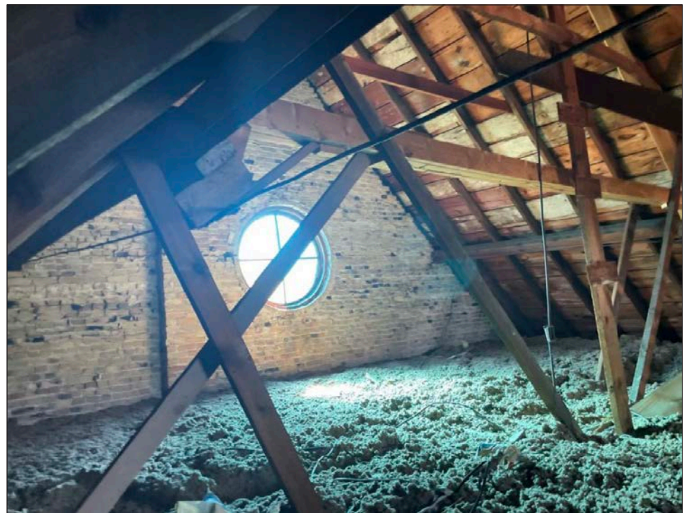
A view of the wood trusses in need of replacement at the old Baptist church.
