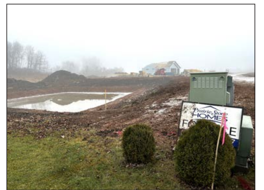
A view of some of the construction underway right now within the Wolf Run Subdivision.
