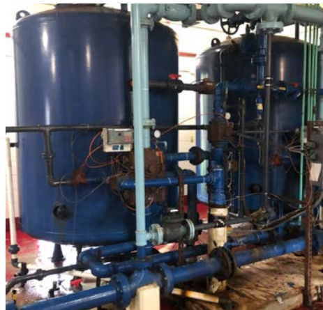
A view of the old water treatment system in Well #2.
